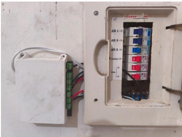
Figure 11. Data collection system installed for energy consumption monitoring.
