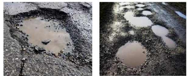
Fig 1: A road image exhibiting potholes
