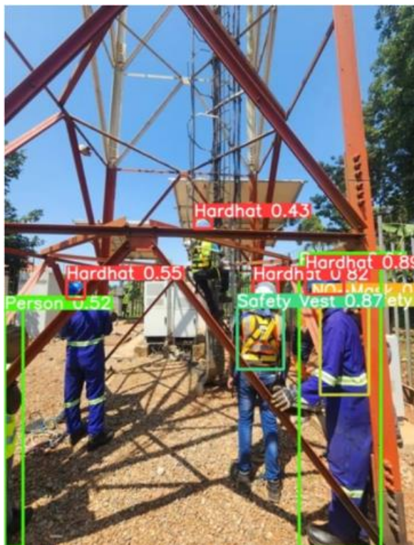
Fig 3: Example of PPE compliance detection in a telecommunication site using YOLOv8
